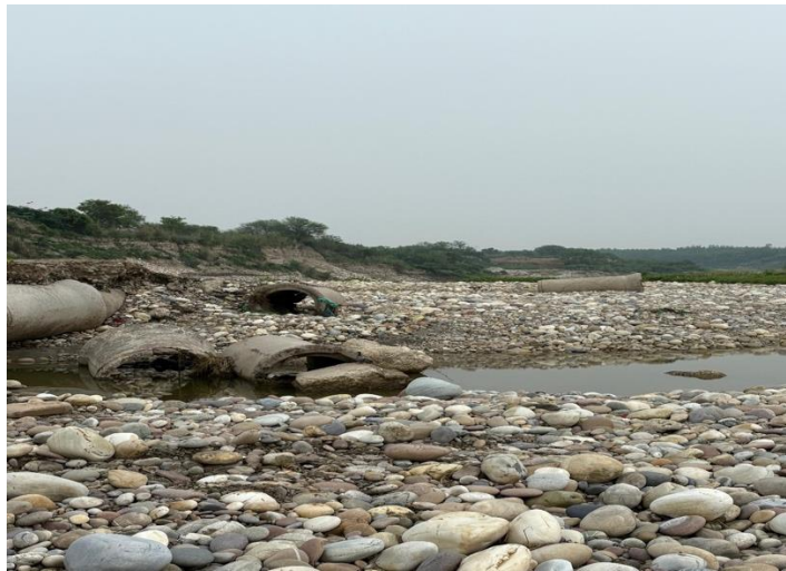
Figure 3.12 Obstruction of flow seen on the river during site visit
